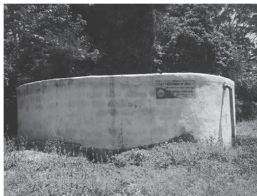
Water reservoir tank
